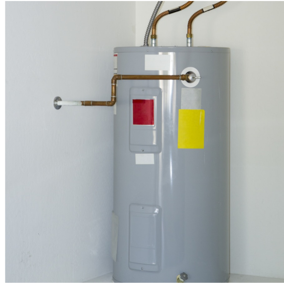
Electric Resistance Storage
